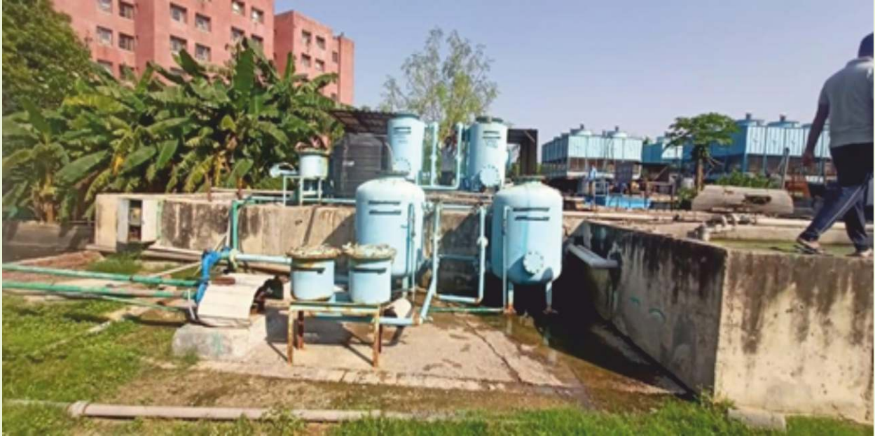
STP Plant at Amity University Haryana
